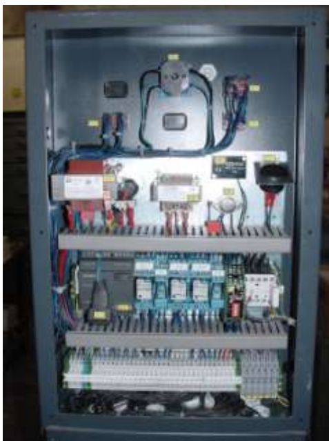
Pic.15 Electrical parts in command unit
